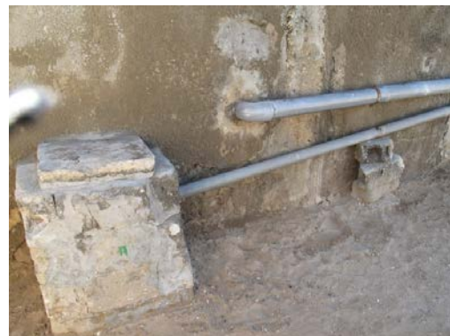
Left: 'Y-shaped' connection used on the ONAS sewer systems in Dakar and Saint-Louis/Darou (source: ONAS). Right: connection via a household connection box in Ngor
