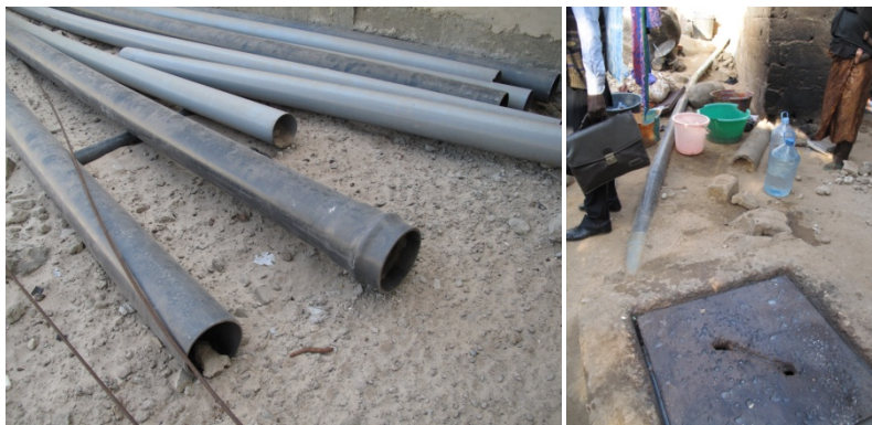
Left: high pressure PVC pipe used for the primary sewers in Cayar. Right: pipes laid on top of bedrock in Baraka, Dakar.
