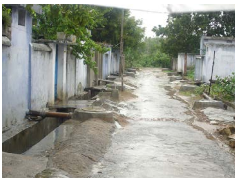
Photograph 1. Simplified sewerage in a resettlement colony in Ramagundam.
