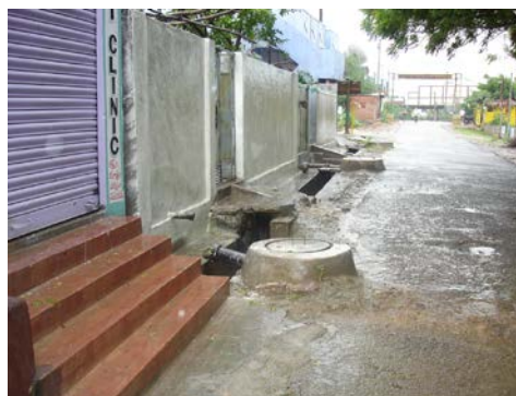
Photograph 2. A shallow chamber for house connection.
