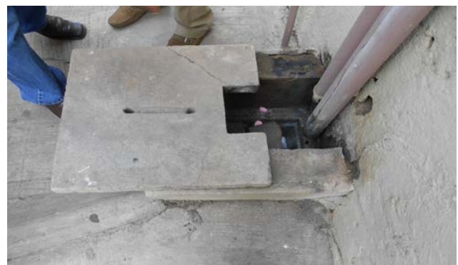
Plate 6: Householders are responsible cleaning of grease-traps.
