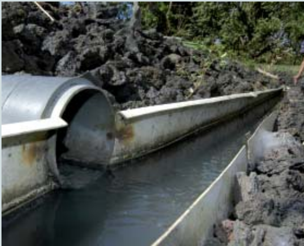
Inlet distribution system at Masaya, Nicaragua. Source: WSP, 2006.
