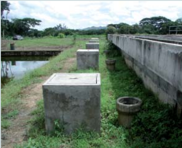
Sludge evacuation system at the Imhoff tank, Masatepe, Nicaragua. Source: Martin Gauss, 2005.
