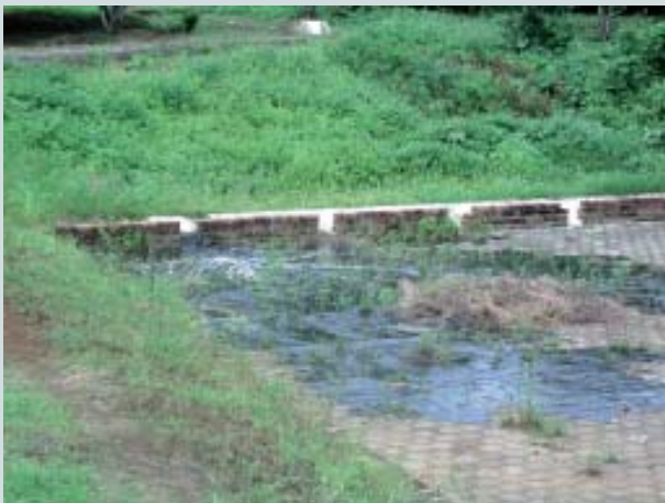
Sludge drying bed at Masatepe, Nicaragua. Source: Martin Gauss, 2005.
