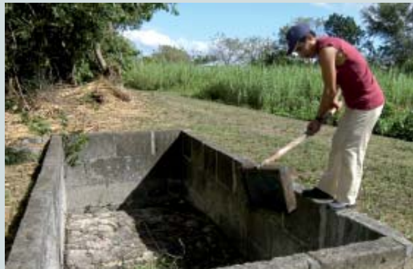
Operator discharging sludge from the grit tank to the drying bed. Source: WSP, 2006.
