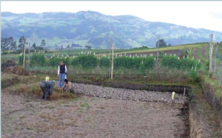
SSHF constructed wetland in Pasto, Colombia, during construction. Source: K. Moncayo, personal communication, 2007.
