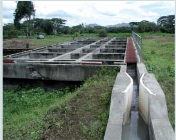
Flow measurement (Parshall channel) and Imhoff tank at the SSHF constructed wetland scheme at Masatepe, Nicaragua. Source: Martin Gauss, 2005.
