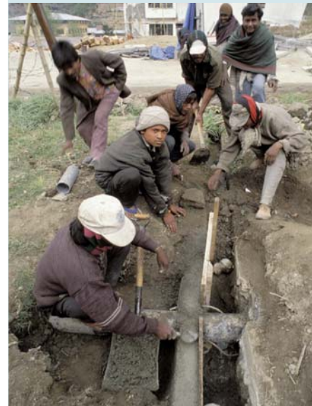
Laying water and sewage lines in Bhutan, a measure that can facilitate access to safe drinking-water and improved sanitation.
