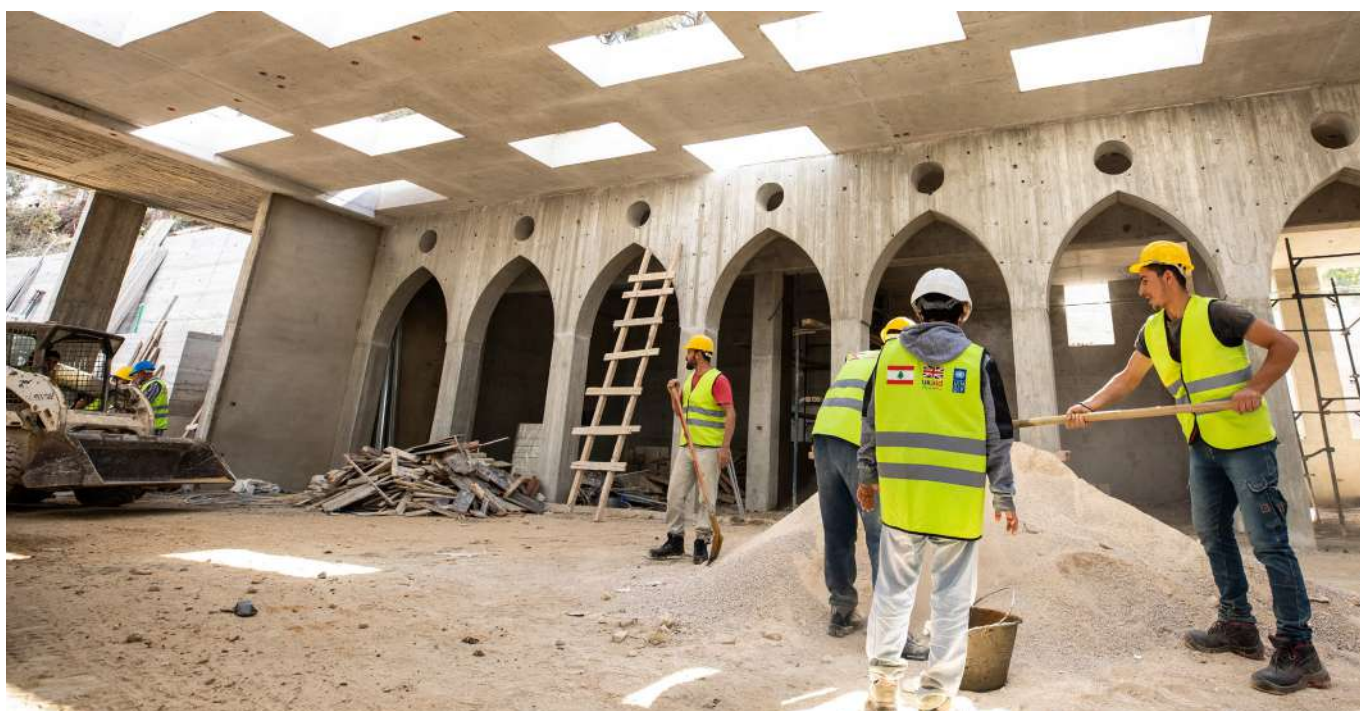
Construction of a Multipurpose Centre for Artisanal Products in Ainab village, Aley, Lebanon - UNDP, 2022
