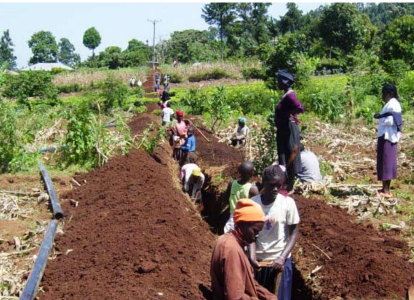
Community participates in the water project by digging trenches for water pipes. Photo © UN-Habitat
