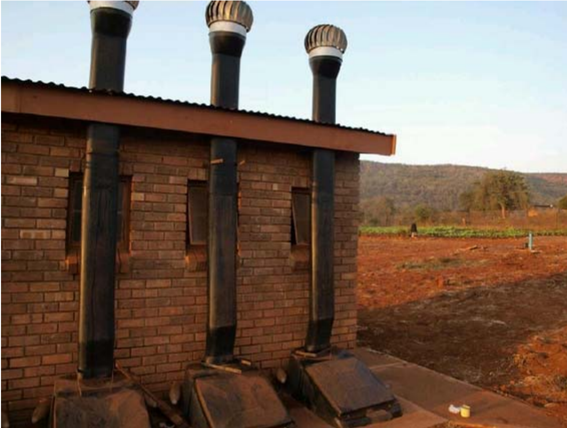
A sample Enviro Loo installation
