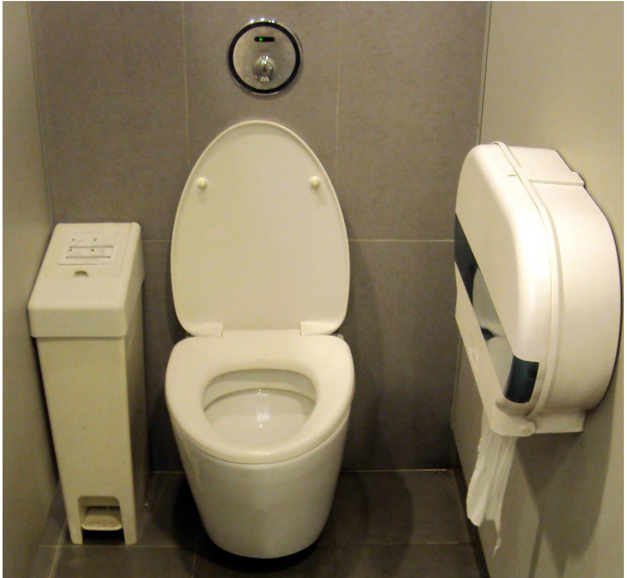
Illustration 17: Wall hung WC with double-roll toilet paper dispenser and foot operated sanitary bin
