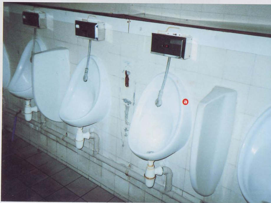
Urinals of inadequate size
