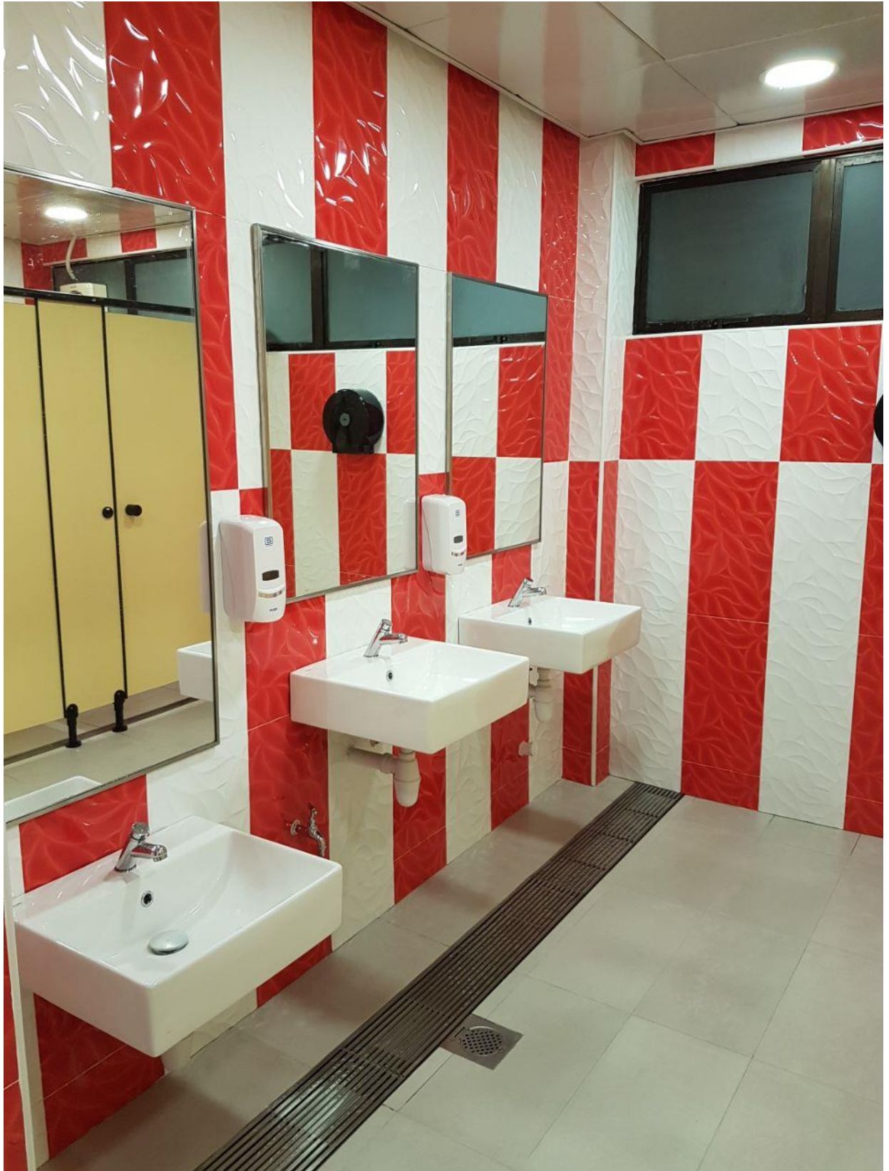
Illustration 15: Standalone wash basins (without vanity tops) and scupper drains with metal grating
