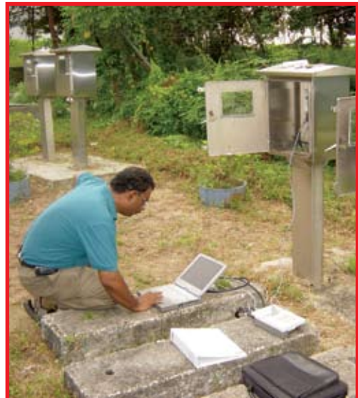
Water utility managers need to accurately measure water produced from the treatment facility. Total water produced is a key input for the water balance.
