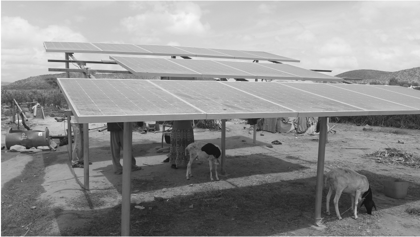
Figure 4.4 Sand on PV modules limiting power output
