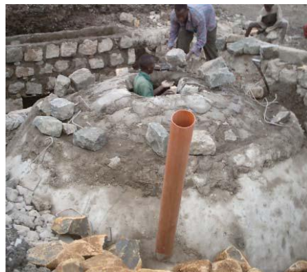
Figure 5: Construction of the Bio-digester chamber (in a fixed dome biogas unit). Photo: Practical
