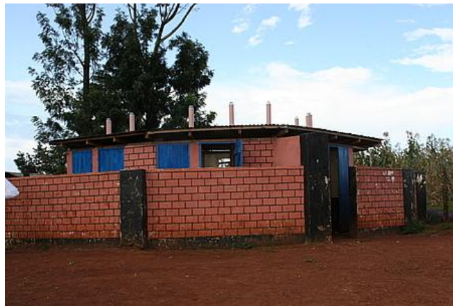
Likhana Primary School, Kitale. Provision of bio-latrines replaced traditional inadequate pit latrines for 908 children who attend the school.
