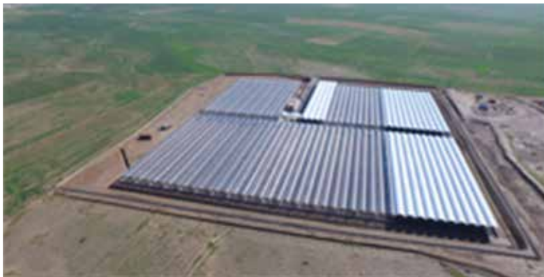
IMAGE 1.1 Solar sludge drying station. SOURCE: RADEEMA.
