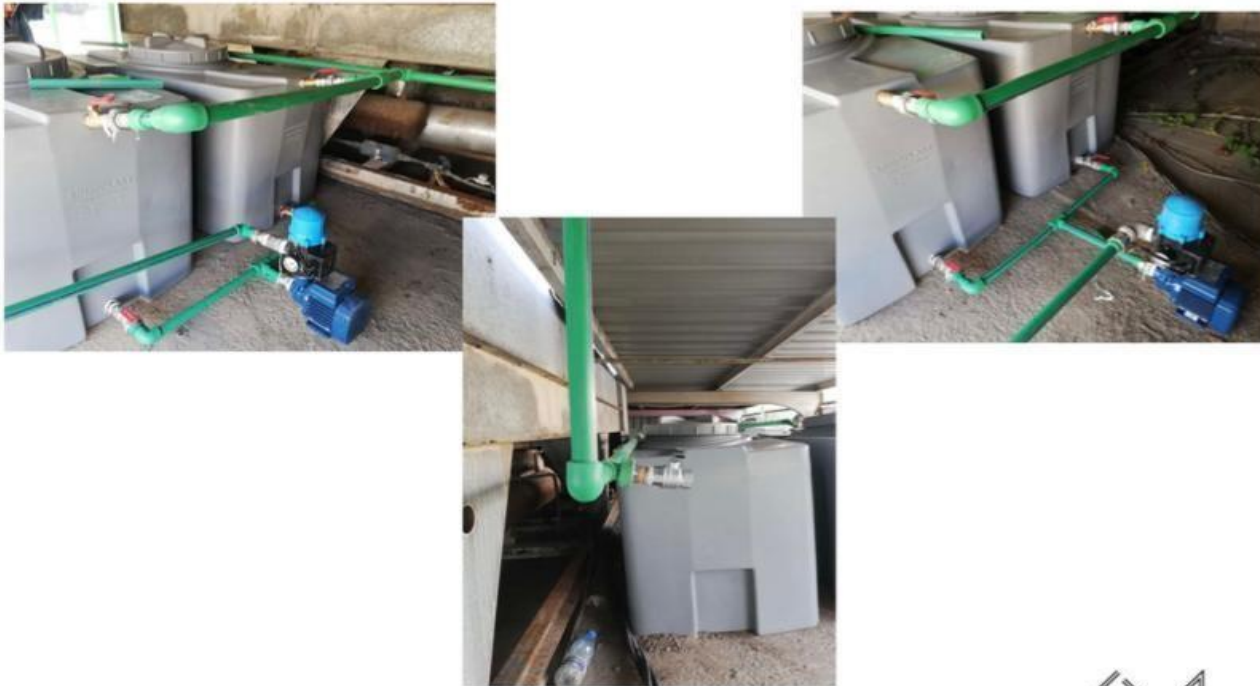
Water Tanks 4 2000L
