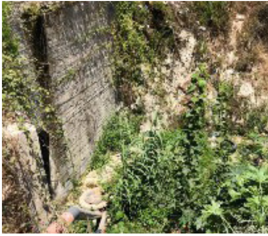
Household Sewage Pipe
