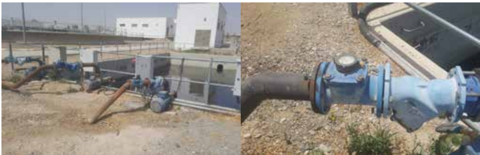
IMAGE 5.3 Effluent storage and irrigation tank and the effluent pumps and the flow meters at Jericho WWTP. Photos: I Abu Seiba.
