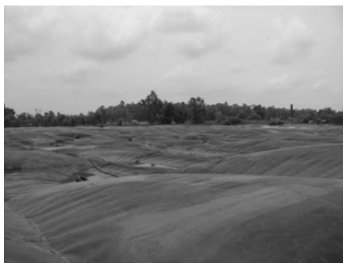
Figure 10.2 Anaerobic baffled reactors (ABR) covered with plastic sheets for wastewater treatment and biogas production
