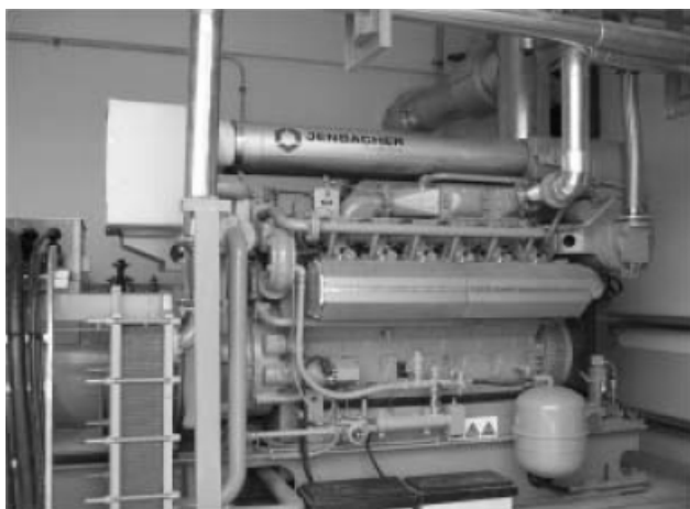
Figure 4.19 Co-generator run on biogas ( www.cogen3.net )
