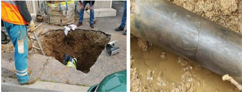
Figure 4.12 Excavation and leaking pipe exposed. (Source: Primayer)
