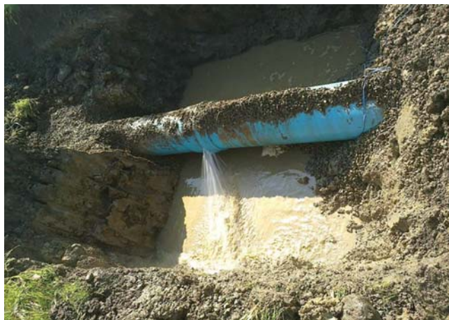
Figure 17.17.4 Detected leak. (Source: Primayer)
