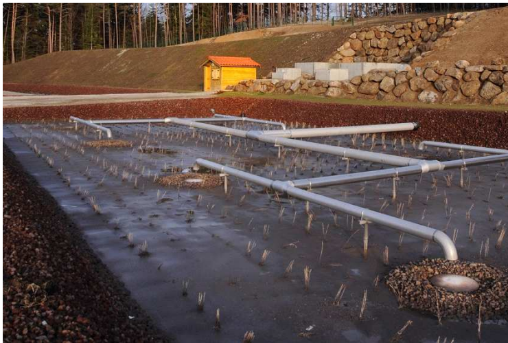
Feeding pipes for the first stage
