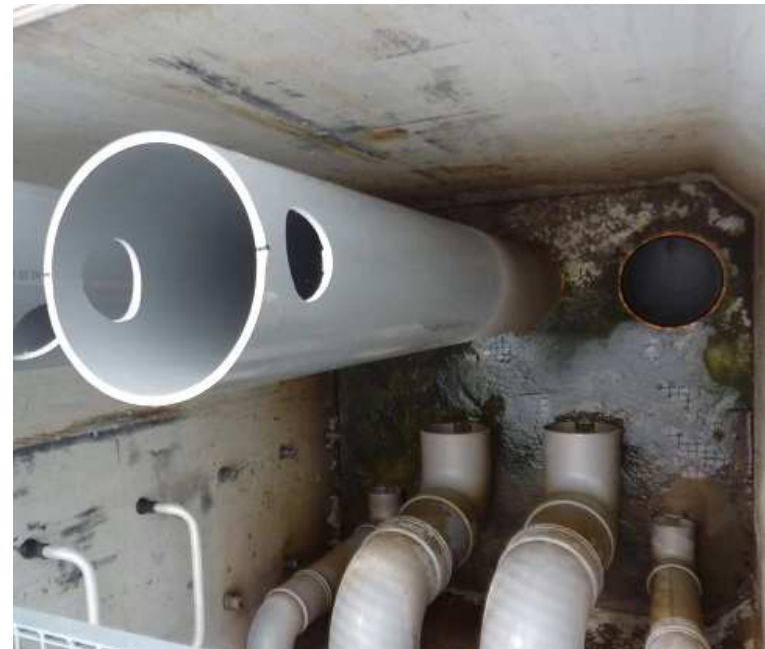
Pipes used as a bung to select the supplied filter
