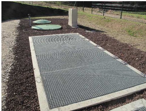
Static grit chamber
