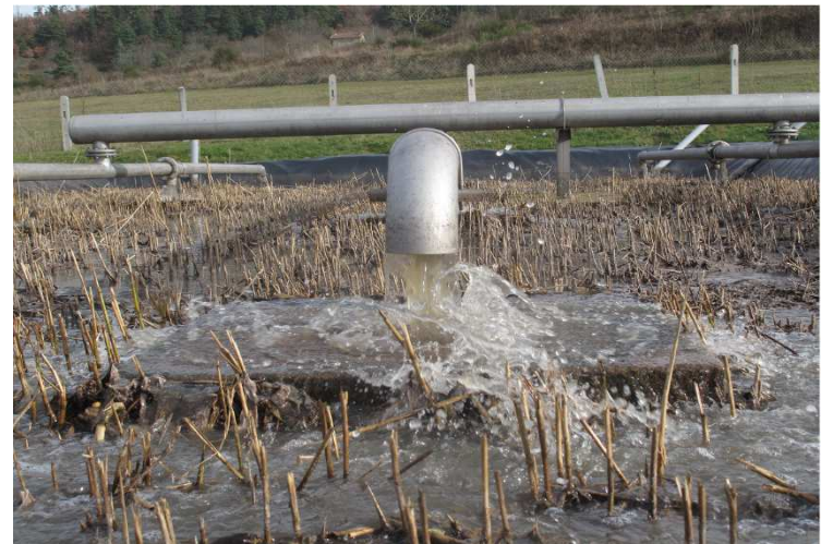
Feeding point and anti-scouring plate
