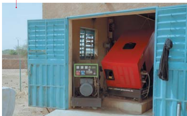
Electricity DSP mini-plant at Keur Massene Source: Joan Bardeletti
