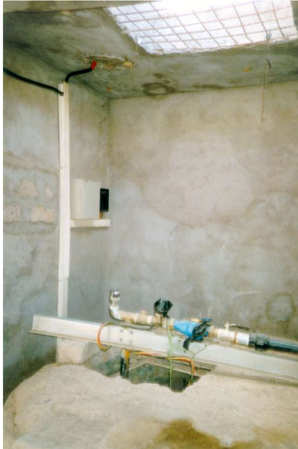
Figure 2. Skylight allowing bird droppings to fall into the well
