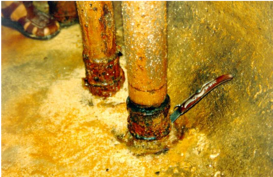
Figure 1. Corroded pipes at the base of a storage tank. Fissures were big enough to accommodate the knife blade.
