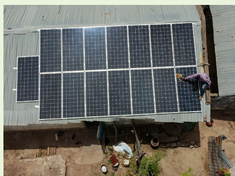
INSTALLATION PV DE SINTHIANG SEYDOU MBAYE
