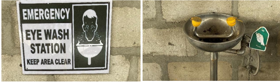
Figure 12: Emergency eye wash station
