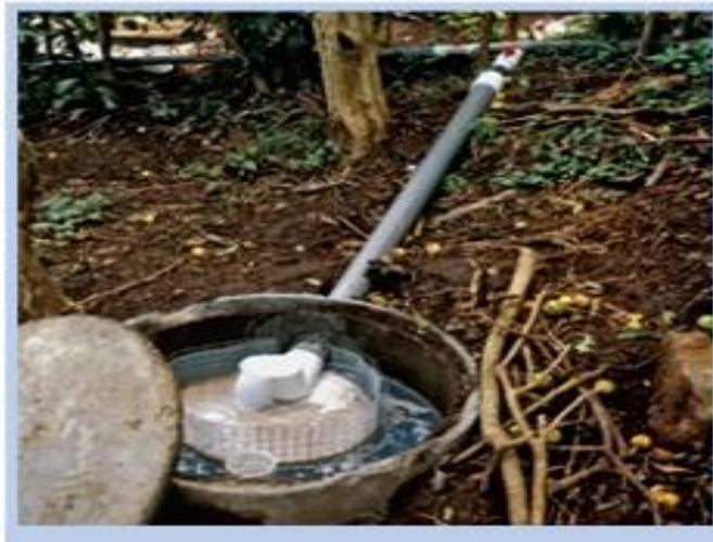
3-7a Settling tank
