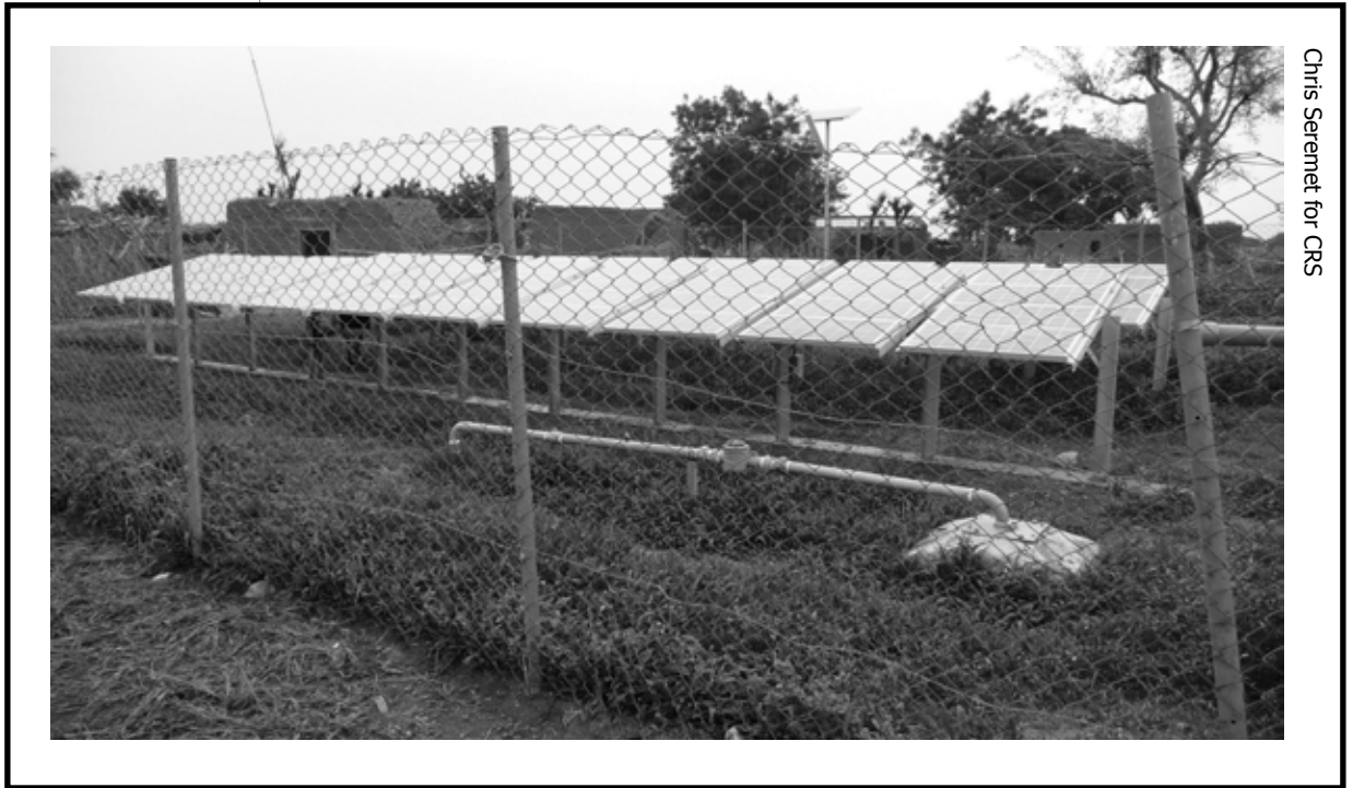
Solar panels supplying power to an electric submersible pump in Mali.
