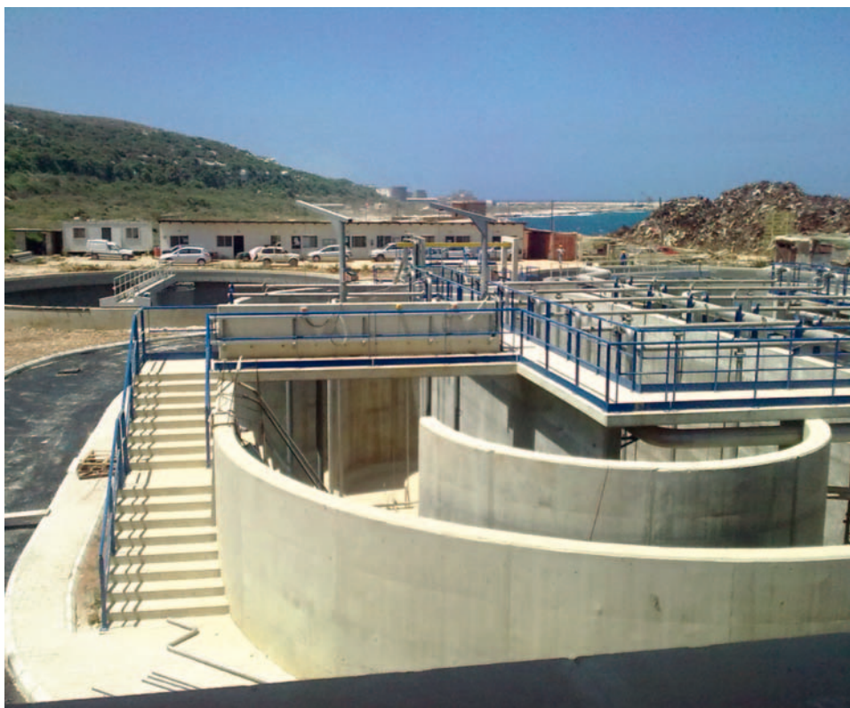
Wastewater installations in the coastal city of Tripoli
