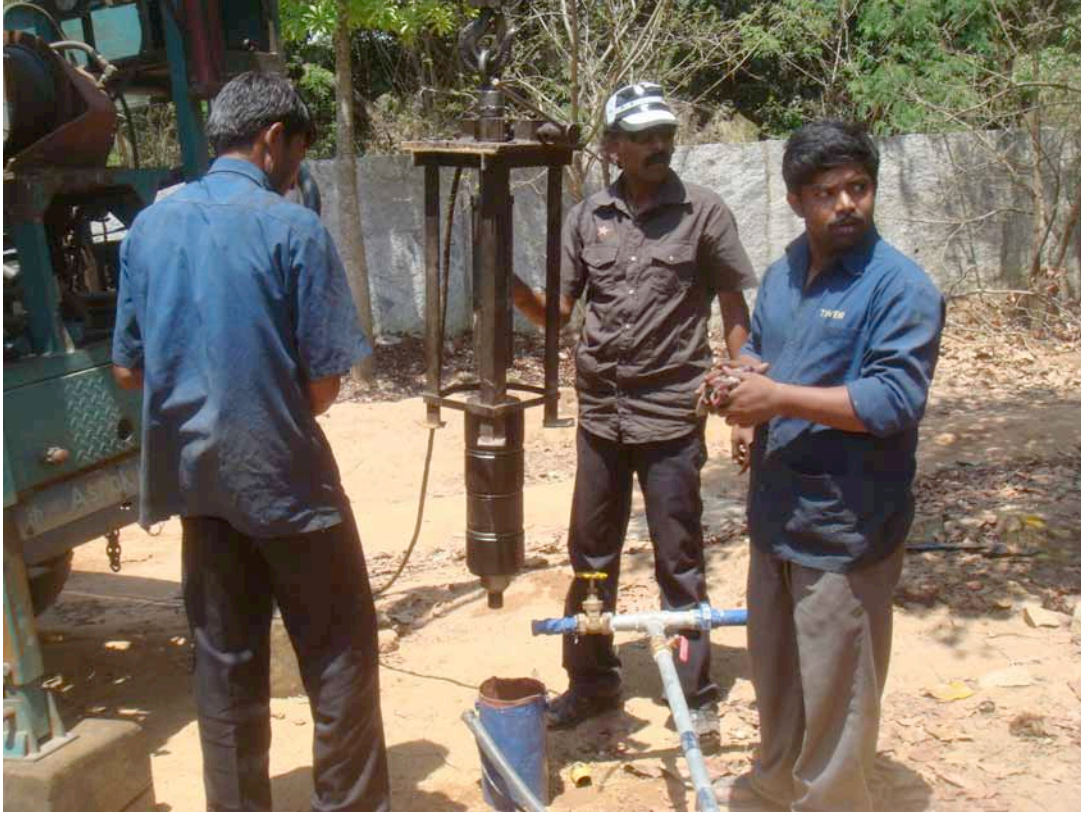
The packer plug with the central pipe for high pressure water being introduced into the bore well
