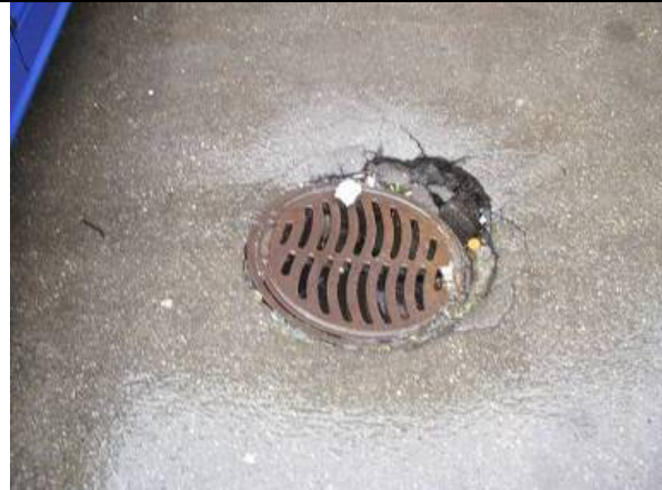
Damage pavement at a floor gully
