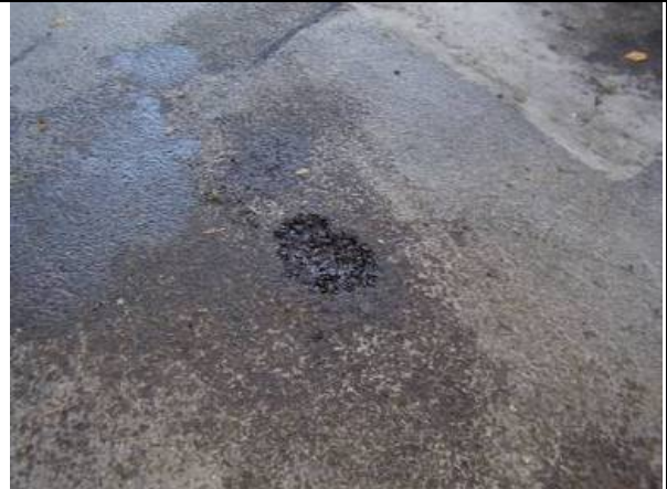
Damaged pavement and oil / fuel spill
