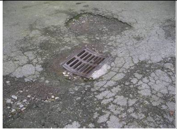
Damage pavement at a floor gully
