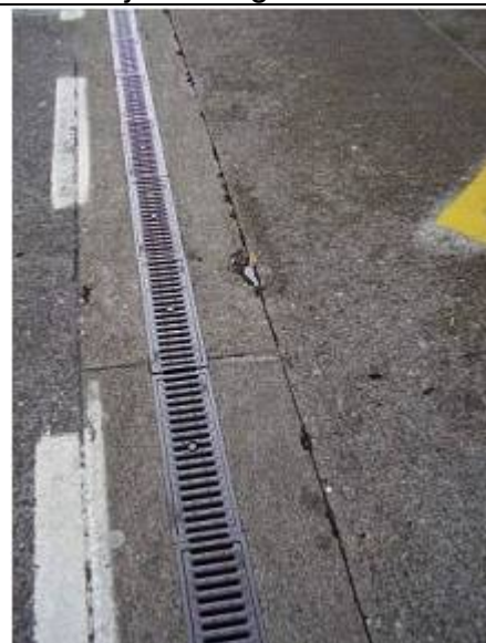
Damaged (leaking) joints along drainage channel
