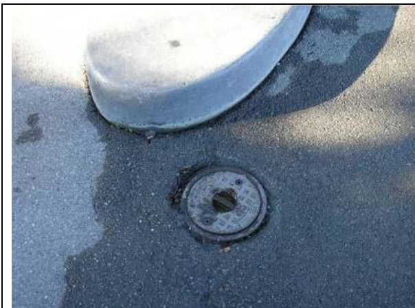
Leaking joint around cover and pedestal
