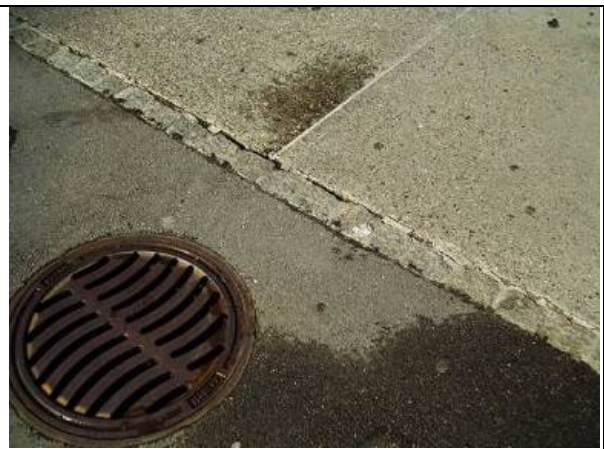
Leaking joints at intersection of different material
