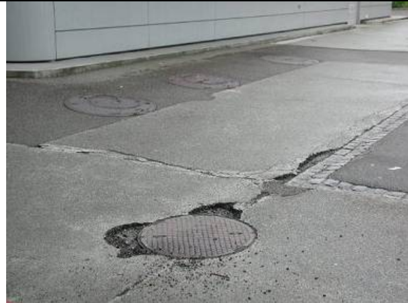
Damaged pavement in filling area
