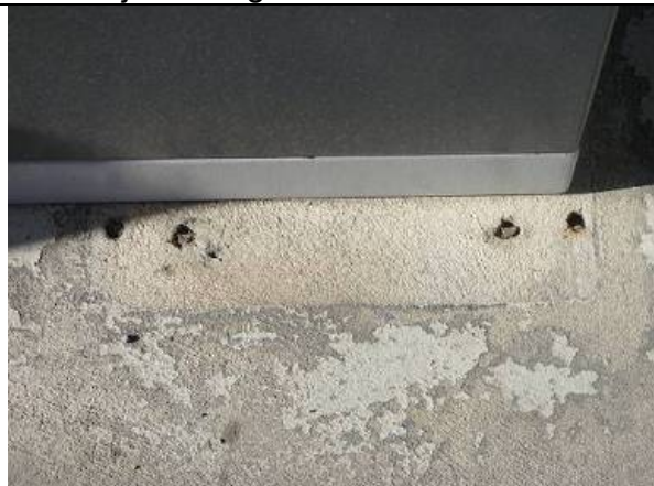
Holes for screw anchor not plugged!
