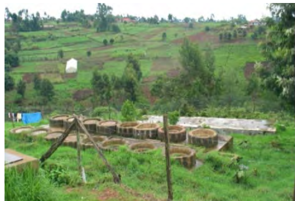
Biogas breeders and digesters at Gachoire Girls Secondary School in Kiambu, Central Kenya, process human waste from the school into biogas for cooking, saving money and trees. ALERTNET/Pius Sawa
