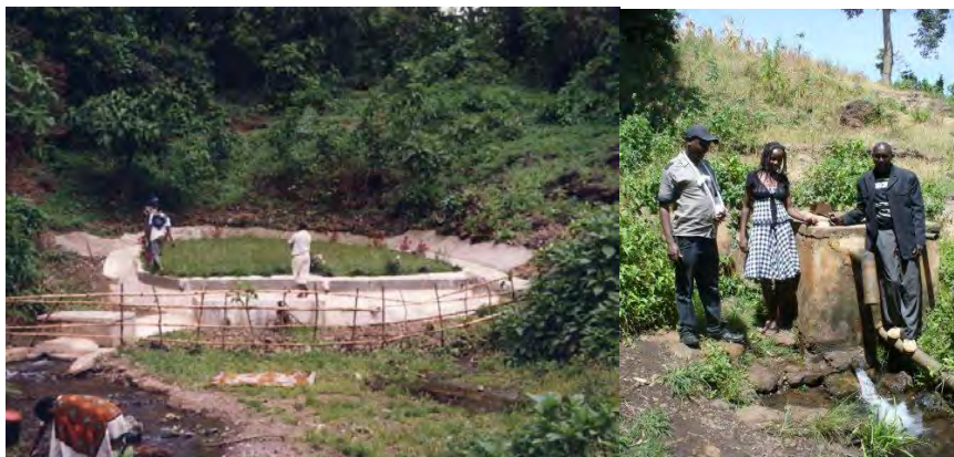
Spring intake and gravity-fed water main SW Tanzania and SE Kenya (Aqua for All)
