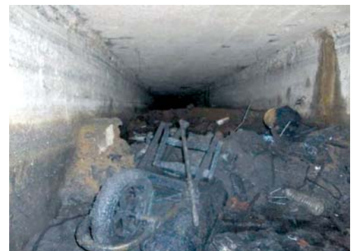
Miscellaneous waste in a sewage collector before cleaning
