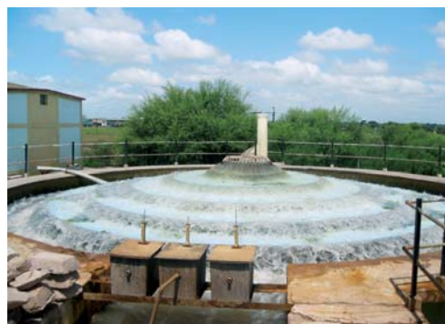
Aeration of Raw Water at Treatment Plant
