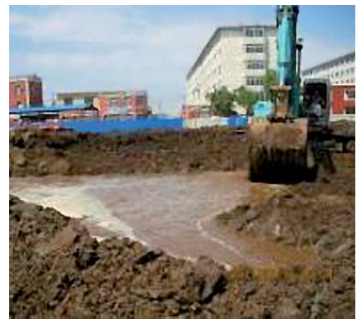
Losses caused by disorderly construction
