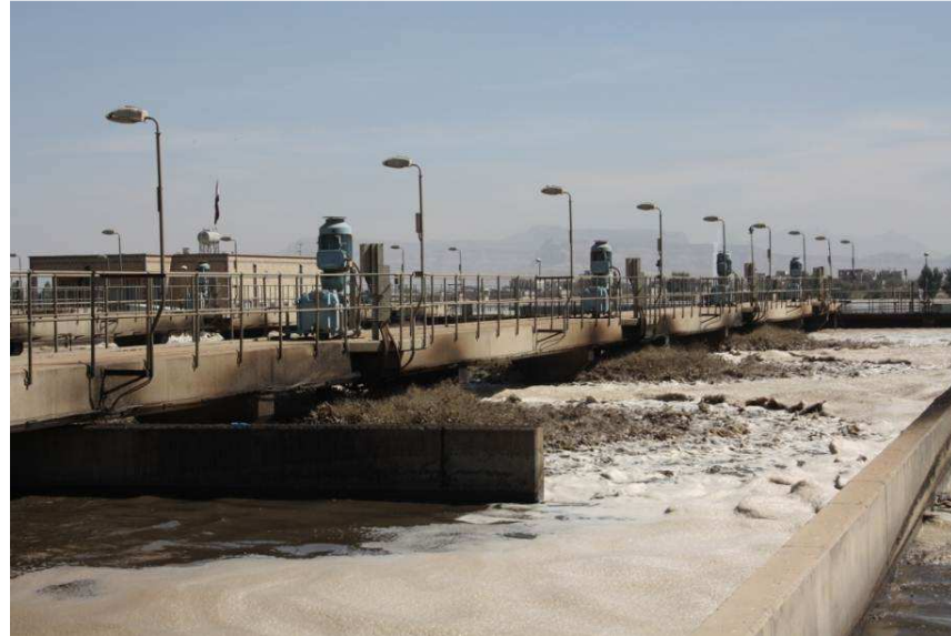
WWTP Sanaa, Aerators
